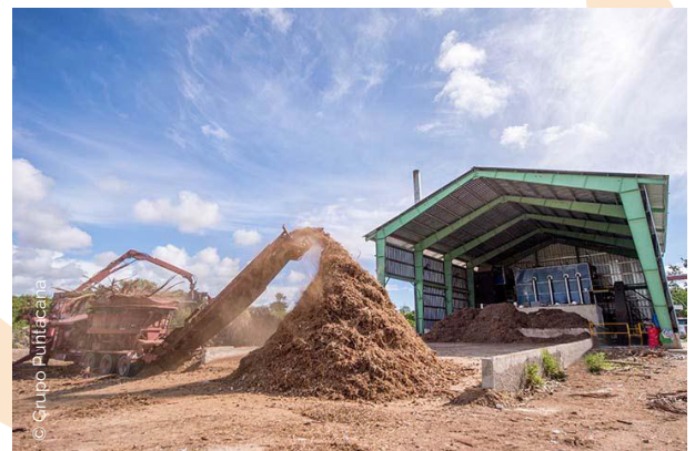
Biomass boiler, at Punta Cana Laundry Service.
