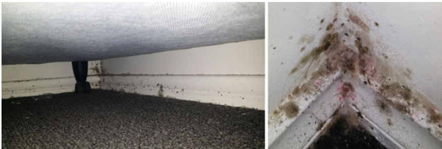
Fig. 20 Under the bed, the wall and carpet have limited exposure to the heating and experience thermal bridging to the external walls
