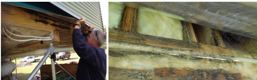
Fig. 5 Often the true effect of condensation happens inside the wall framing. A builder helps dismantle the sheet metal cladding that is hard fixed against the studs (no battens) causing the wrap to be thermally bridged with the cold exterior. Indoor vapour, unable to pass through the foil wrap condenses on the insulation which acts as a reservoir, keeping the studs and bottom plate a moist breeding ground for mould
