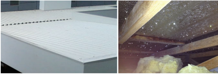
Fig. 13 The constantly wet, and often dripping underside of the roof
