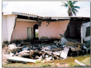
Hurricane damage (Republic of Honduras) Photo: AYUda a Centro America (AYUCA), a non-governmental organization (NGO)
