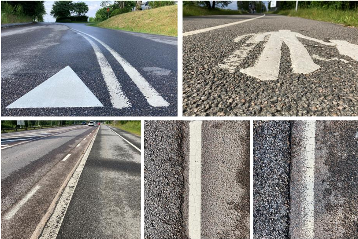
Figure 6. Thermoplastic road markings with varying degrees of wear. Photo: Delilah Lithner.
