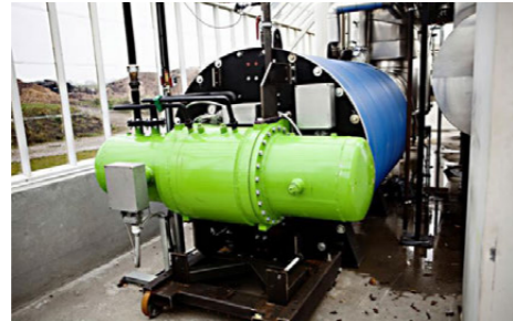
Energy From Waste Pyrolysis Plant
