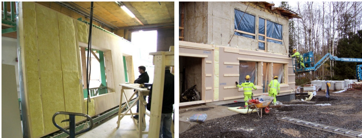
Figure 13: TES element prefabrication in Haapavesi and assembly on site (photos M3 Architects, 2012)
