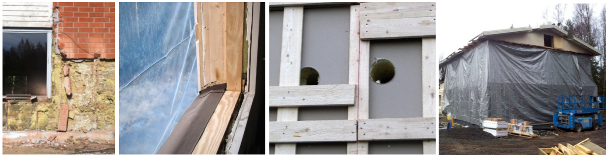
Figure 15: Critical site details: partial demolition, window sill sealing, ventilation penetrations, rain protection (S. le Roux). Site management quality is needed to respond appropriately to existing conditions, maintain site waste management, ensure structural integrity, deliver good air tightness and moisture control, and accurately assemble and protect retrofit components.
