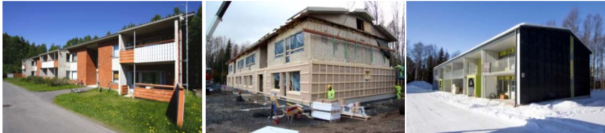
Figure 30: Oulu demonstration project in 2011, TES assembly phase in 2012, and completed in 2013 (photos M3 Architects)
