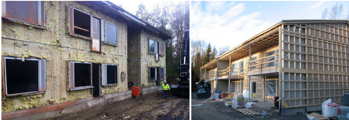
Figure 12: Removal of the external layer of precast concrete sandwich elements in September 2012, and completed assembly in November 2012 of prefabricated timber facade elements, concrete balconies with steel supports, and a new roof assembled on site and lifted into place in 4 large sections (photos S. le Roux, September and November 2012).
