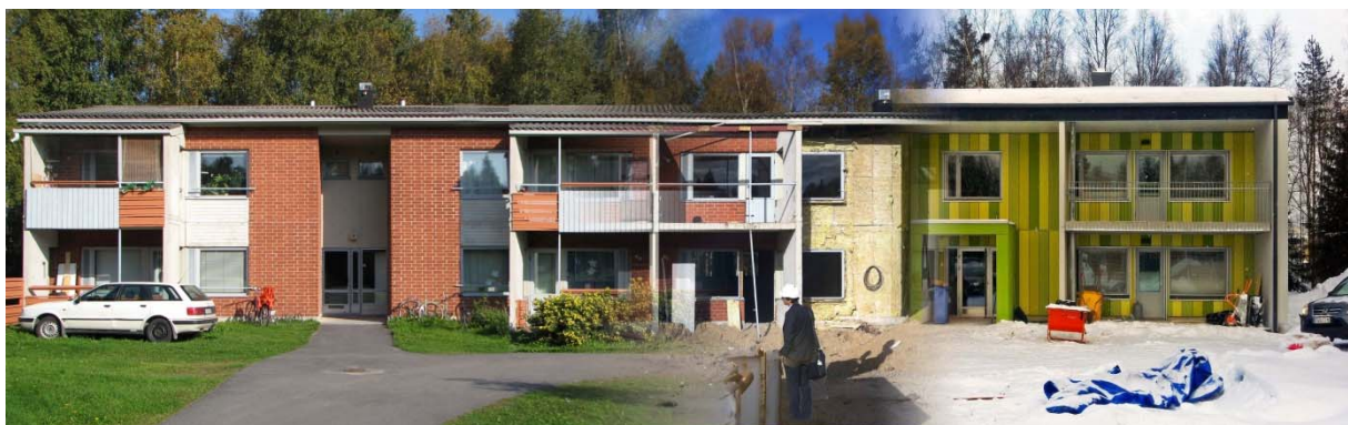
Figure 9: Retrofit process collage. From left: original state 2011, demolition phase 2012, and finishing off 2013 (S. le Roux)
